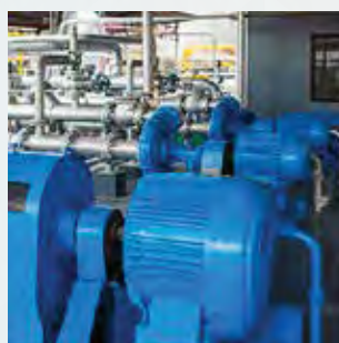
Pumps (Electrical & Pneumatic)
