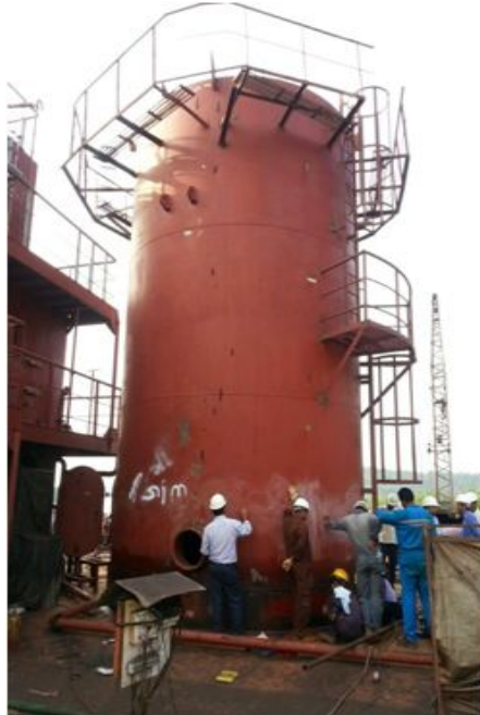
23 mtr. ht. Crane Pedestal with a Dia of 5 m / 45 mm thickness plate
