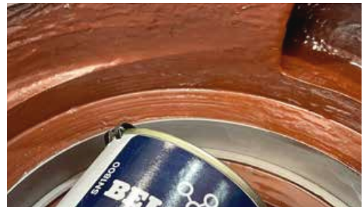
Disappointing repair reality – brushed-on epoxy ceramic. No engineer wants to see such turbulence-generating results anymore. Today, “good” looks fully different ...
